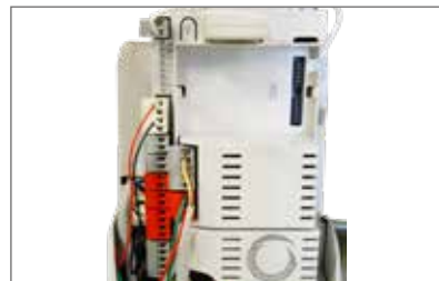
Control board 14A
