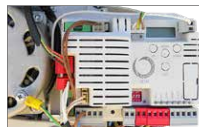
CT102 control board
